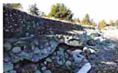
Erosion along seawalls
